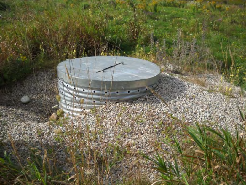
SWM Facility No. 96 Outlet
