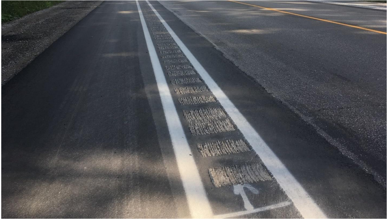
Figure 3 Bike lane on Victoria Road in Guelph which has a painted buffer with rumble strips set into it.
